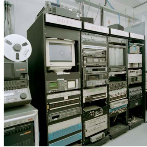
Fig 3. Control and Switching Room Equipment to display images in the ATEL Viewing Room
