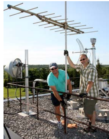
Fig 7. Installation of an 8-VSB Gap-Filler transmitter
